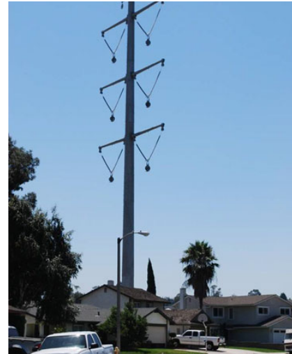
Figure 1 Chino Hills Transmission Tower
